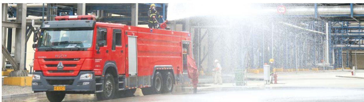
Xinjiang GCL polycrystalline silicon purification project 113B -A rough separation tower hand valve front flange leakage drill
